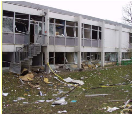
Figure 2 – Example of overpressure damages in the building No 2 located at 50 m in the front of the building No 5, source of the explosion (Neunlist, 2007).
