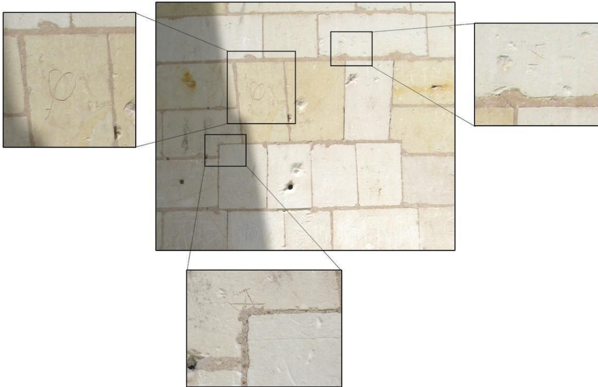
Fig. 2: South façade: door walled on the first left span, with a lapidary sign cut by the addition of a stone to the wall above the door, probably before 1555
