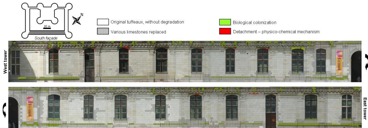
Fig. 8: Age and decay features of stones in the south façade
