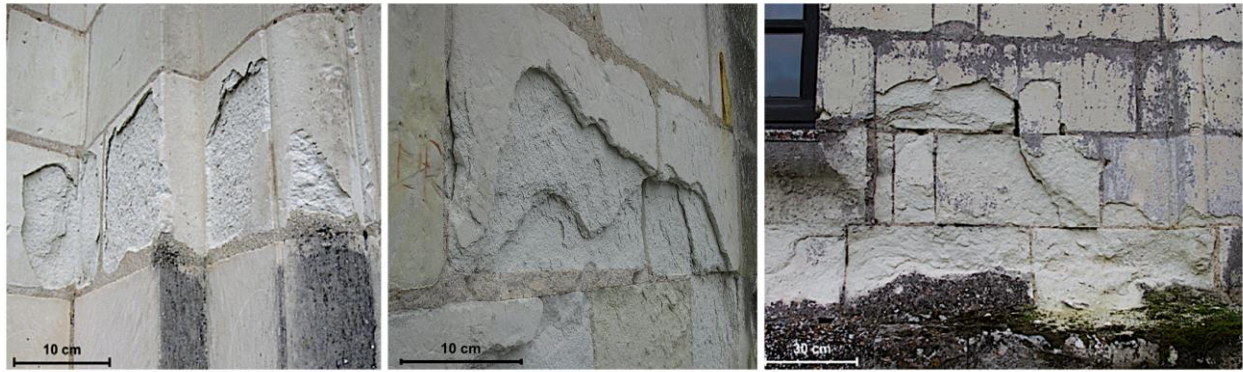
Figure 1. Examples of stone spalling at the Castle of Chambord
