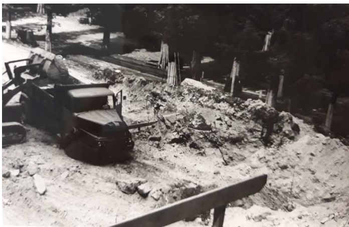
Fig. 13: Start of the work to set up the ionizing radiation building BIPM Archive
