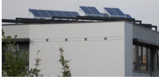
Figure 4. PV installation of the Centre Pierre Guillaumat of UTC [12].
