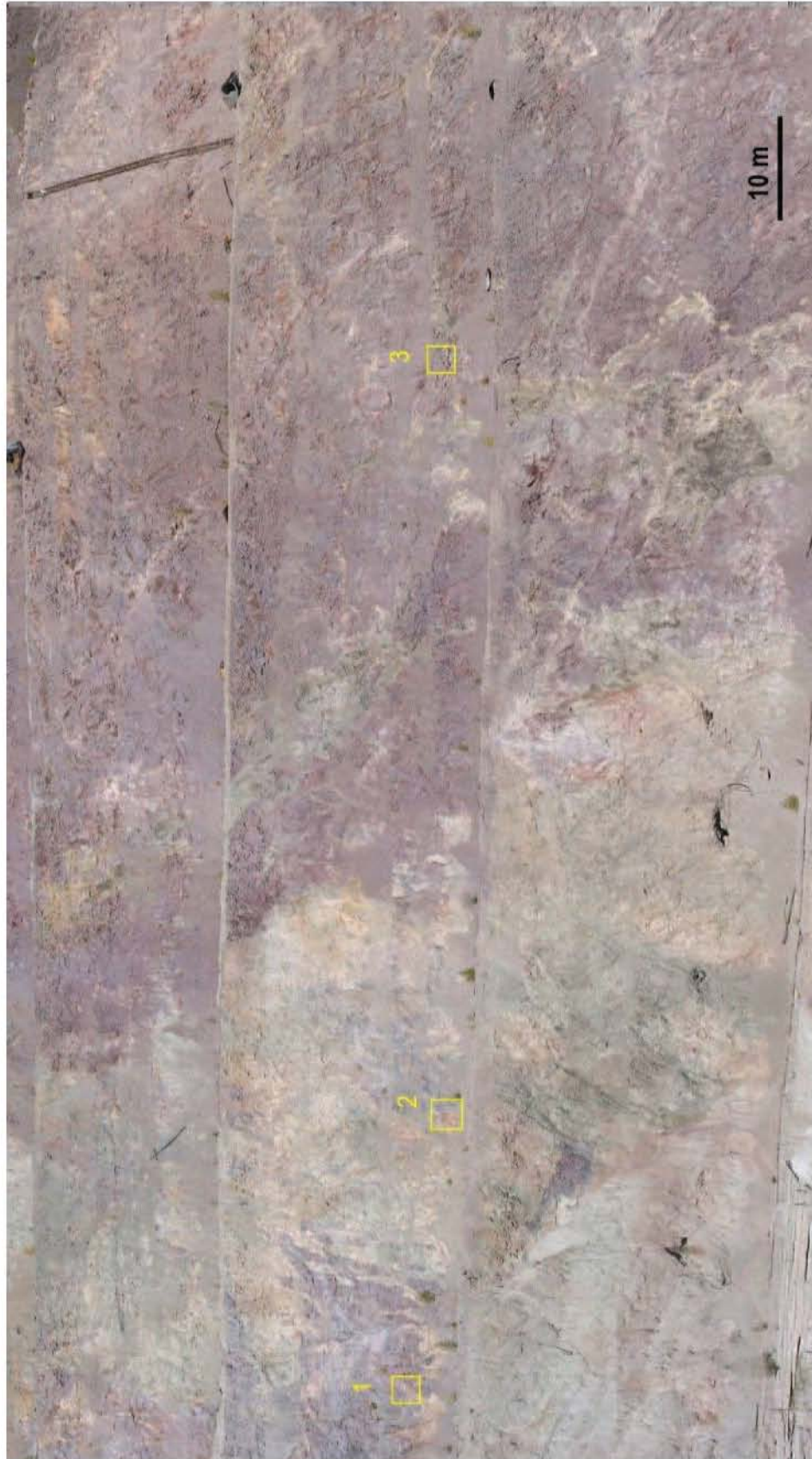
Fig. 2.6. Halos of preore and postore alteration in trachydacites in the west-northern wall of the Tulukui open pit. Weak preore alteration is presented by brownish-red dacites while postore alteration is manifested as intensively bleached light greenish-grey and orange dacites. Rectangles with numbers – areas of detailing: 1 – Fig. 2.7 and 2.8, 2 – Fig. 2.9, 3 – Fig. 2.10.
