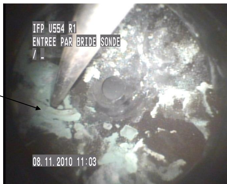
Figure 6.19: Visual inspection of the reactor interior by use of an endoscope at the end of the experimental tests.
