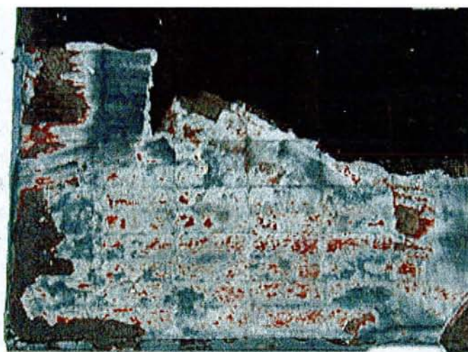
Figure 87: Picture of the separator from the AJS 80 kPa battery with some rest positive active material on the top part and the thin corrosion layer in white
