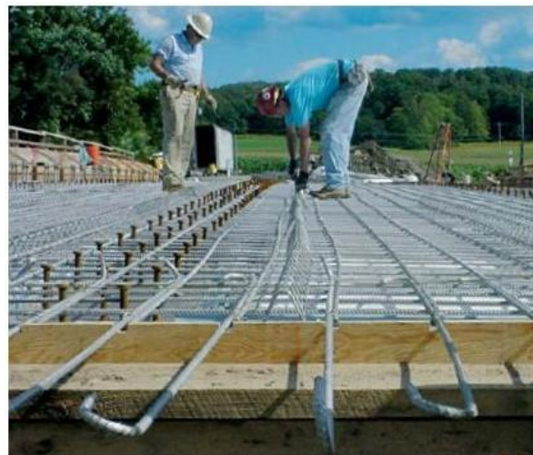
Fig. 2. 4 Installation of inoxydable steel rebar at the French Creek Bridge, Chautauqua Co., NY [22].
