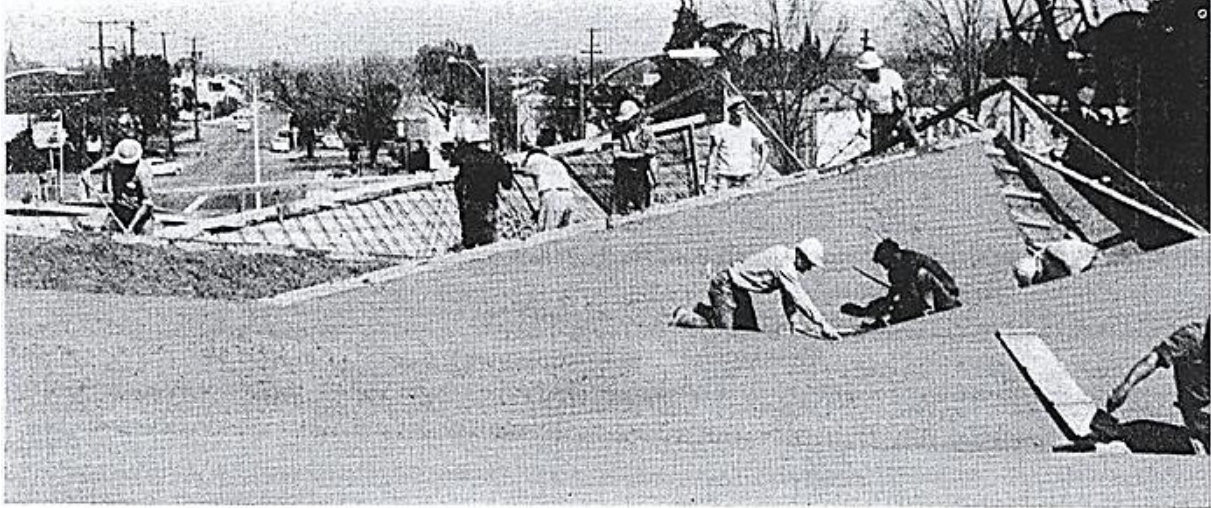
PEAKED ROOF. Workmen put the finishing touches on the Yuba City, Calif., Bank's peaked roof, the first application of ChemComp expansive cement
