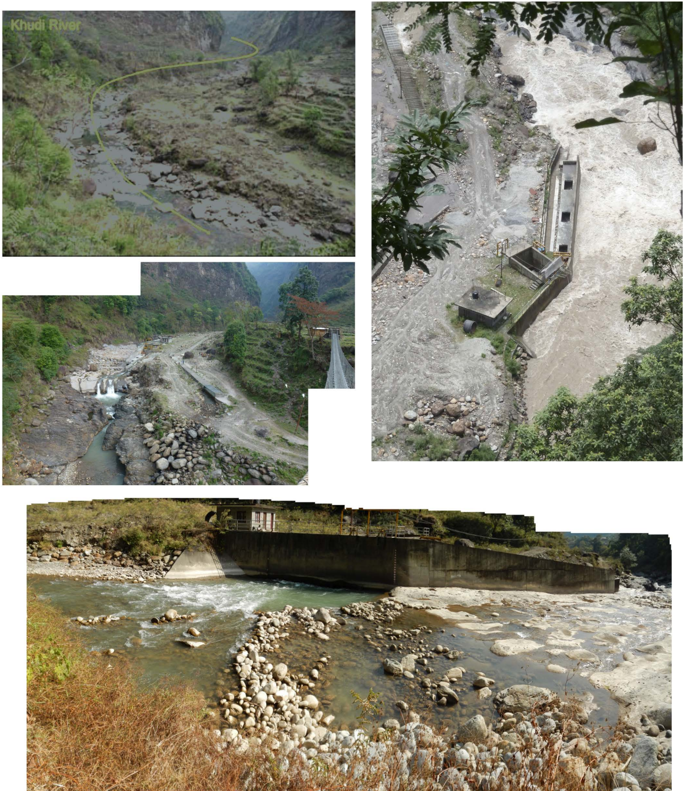
Figure B1: Intake setting constituted by a vertical wall on the Khudi left bank, a concrete weir and ramp and a boulder evacuation channel down to the base of the ramp. Top left pictures were taken from below the structure and offer a view on the Khudi river before (Shrestha and Phuyal, 2006) and after intake dam completion. The
