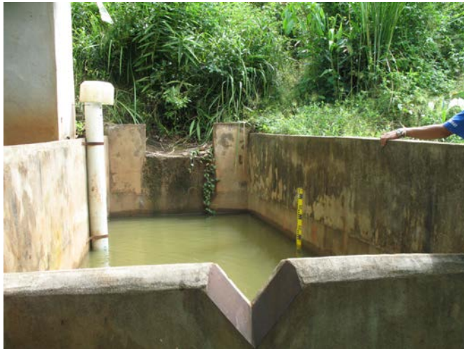
(a) La station S7
