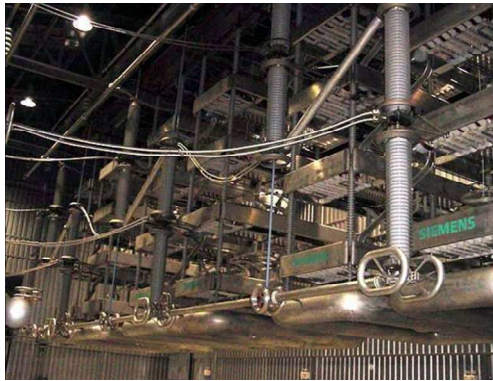
a) Thyristor converter valves
