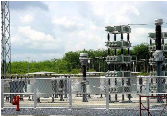
a) AC filters and shunt capacitors
