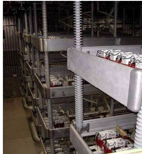
d) Insulator structure
