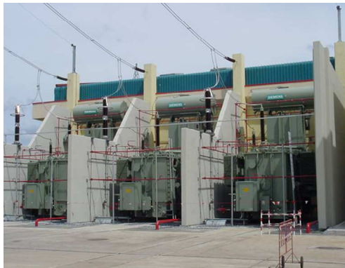
a) Converter transformer station
