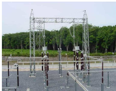
c) DC switchyard
