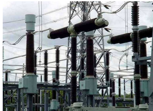
d) Circuits breakers
