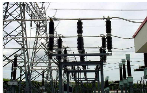
f) Disconnecting switches
