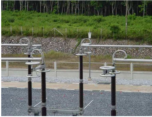
a) Disconnecting switches
