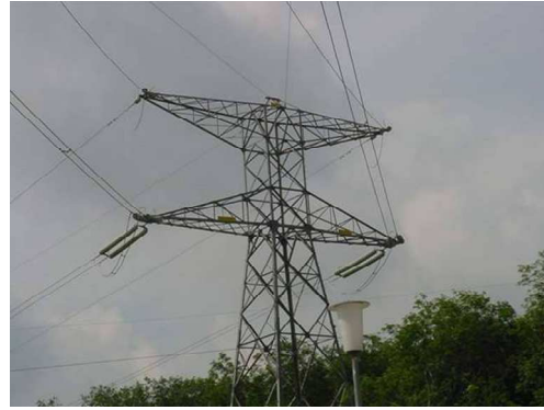
b) 300 kV, 300 MW DC Transmission line
