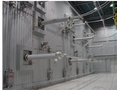
b) Converter transformer inside valve hall station
