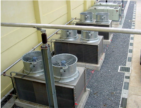
c) Valve cooling system b-Station
