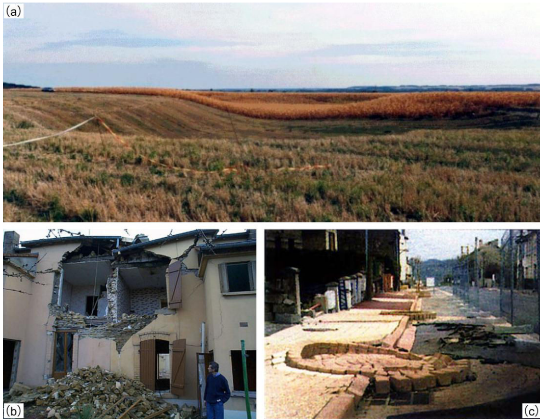
Figure 3. Subsidence phenomena in Lorraine: (a) farmland (source: INERIS); (b) building (source: GISOS); (c) road (source: INERIS)
