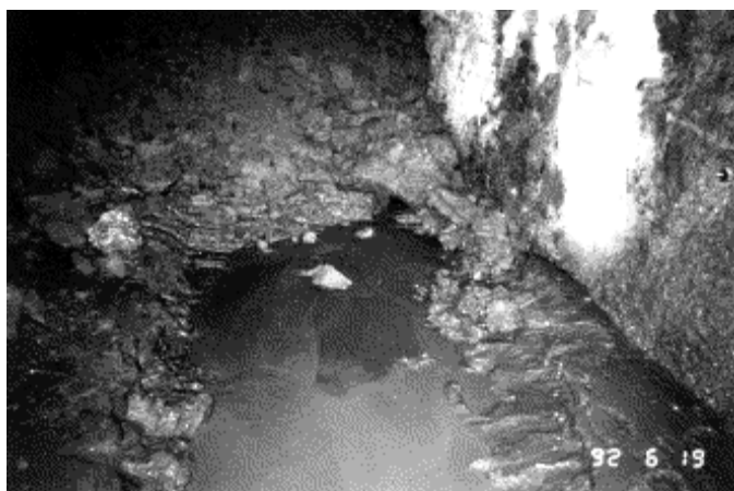
Figure 10. Inondation du tunnel de Wushantou, Japon 1992, (Wanget al., 2002)
