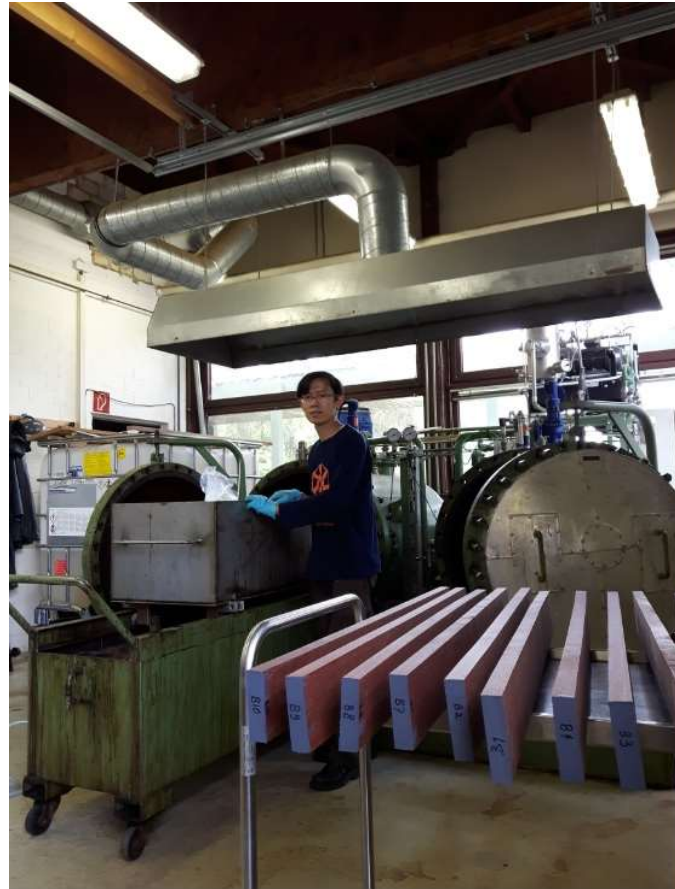
Figure 35: Vacuum-pressure impregnation chambers during up-scaling, Wood Biology and Wood Technology, Göttingen University, 2018
