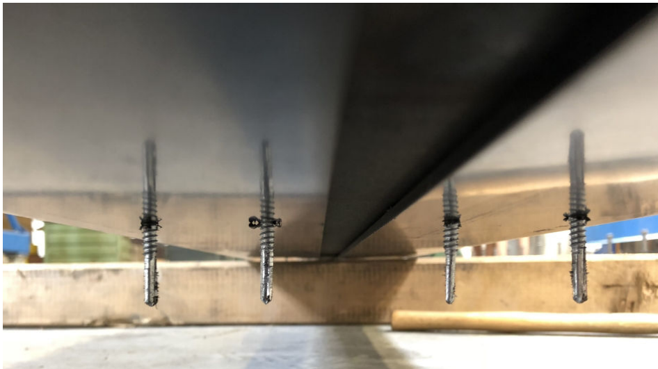
Figure 4.5 – The self-drilling screws in the “wrong” direction before being cut
