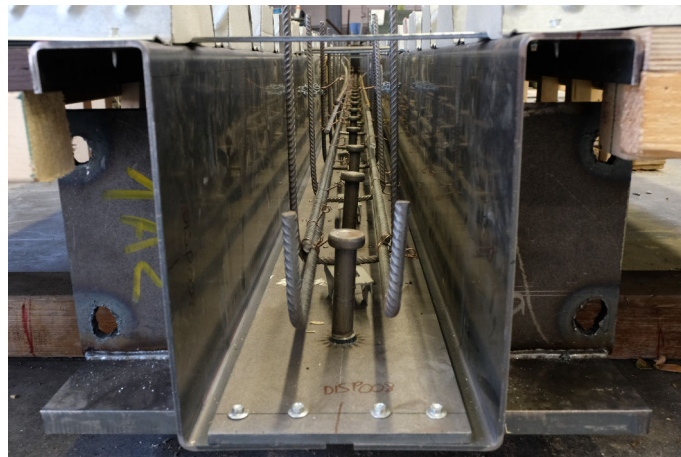
(b) Local view around the studs
