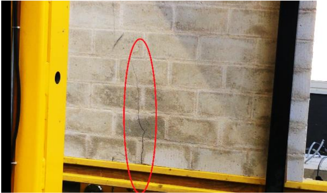
Fig. VIII.14. Cracks appearing in the wall.
