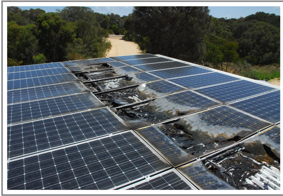
Figure A.6. Arc Fault damage in a 10 kW installation, due to inappropriate AF handling.
