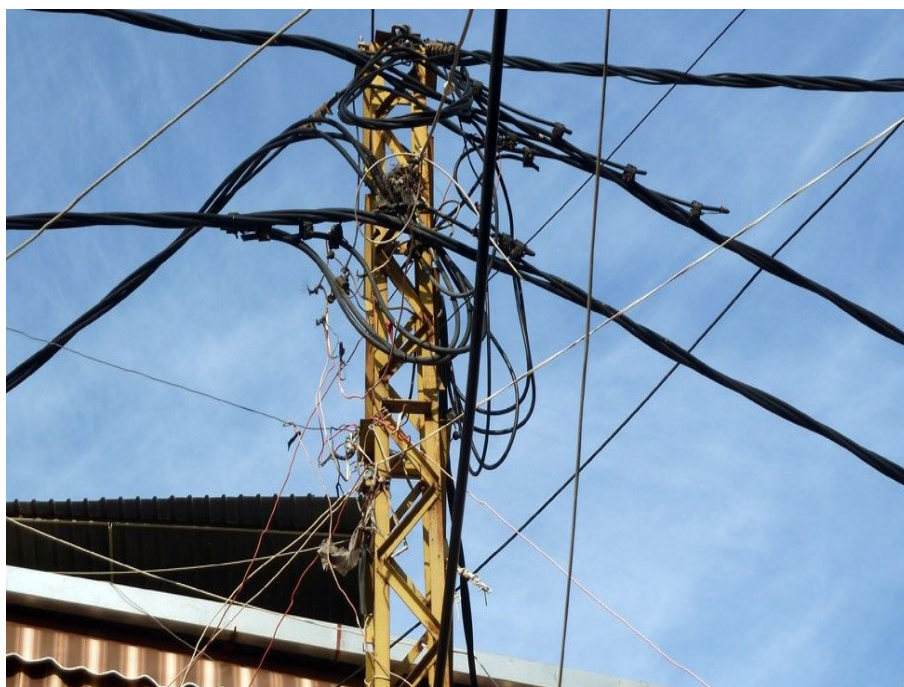
Figure 24: example of illegal connection on the EDL's grid (Ref. BBC, Dec 2019)
