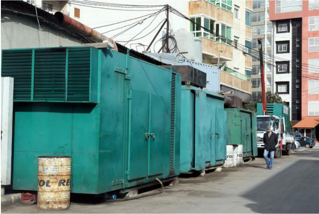
Figure 17: DG network installed between building in Lebanon (Reuters 2019)
