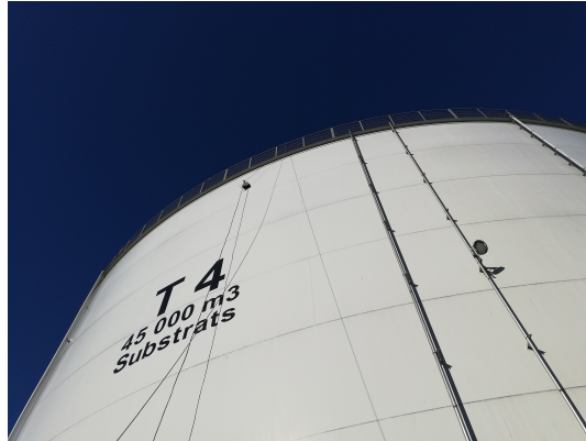
Figure 1.2: The Altiscan crawler navigating on the facade of a 20 m high storage tank.
