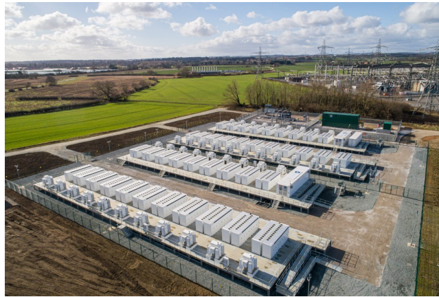
FIGURE 6 – An example of Battery energy storage systems site, from [19]
